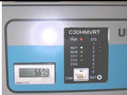
Figure 5-2 Ready for operation
