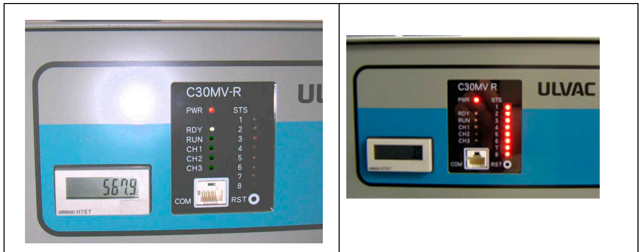
Figure 5-2 Ready for operation (left)
