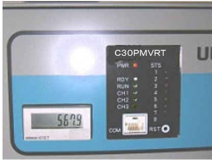
Figure 5-3 Ready for operation
