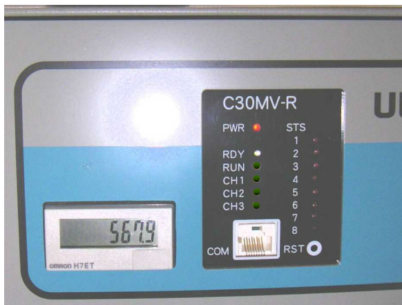
Figure 5-2 Ready for operation
